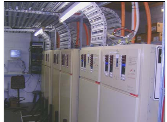
The "Old" dimmer cabinets— installed circa 1983
