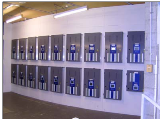
EKO Dimmers now installed and running prior to final coat of paint.
