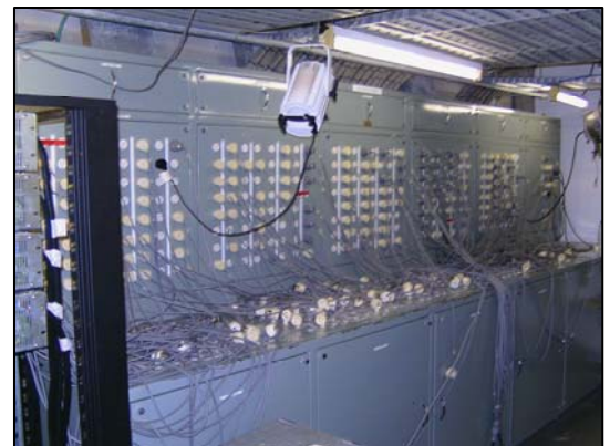
The labour intensive cable patch system
